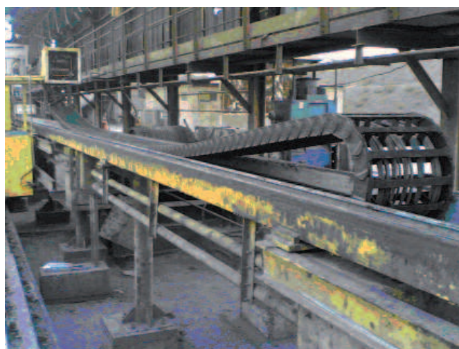
Picture PM0409-03: igus GmbH, Cologne Rough conditions in the steelworks in Isfahan (Iran). Because the heavy steel chain used before did not work, it has now been replaced by a slimmer and lubricant-free plastic energy chain from igus.
