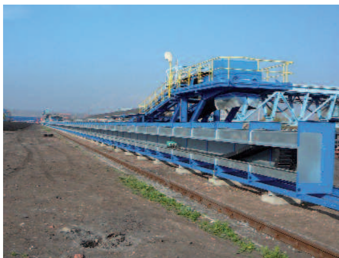
Picture PM0409-02: igus GmbH, Cologne Roller energy chains from igus reduce the friction factor and thus drive power. The photo shows the longest plastic energy chain in the world, a 615 m in the lignite-fired power plant in Tusimice/Czech Republic.
